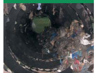
Drum screen interior view
