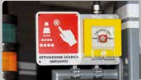
Fire extinguish system
